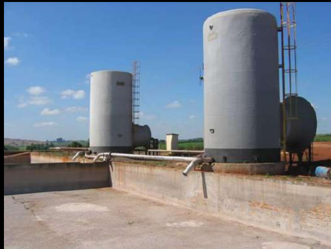
Vinasse cooling and reservoir coated
